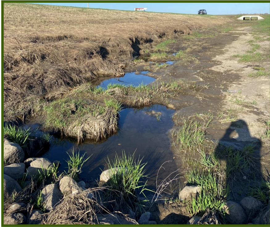
Exhibit 1 - Drain 4 Bank Failure
