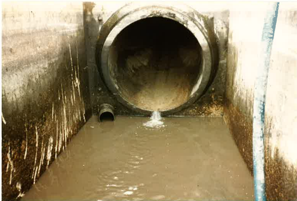
Photo No. 8 - Shale Removal Complete. Note view of Drawdown Pipe adjacent to Conduit.
