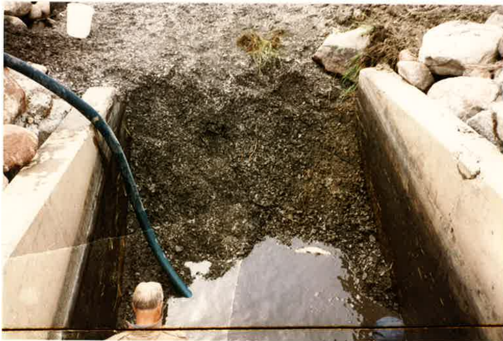
Photo No. 2 - View of Stilling Basin after most of the shale had been removed the morning of July 16th.
