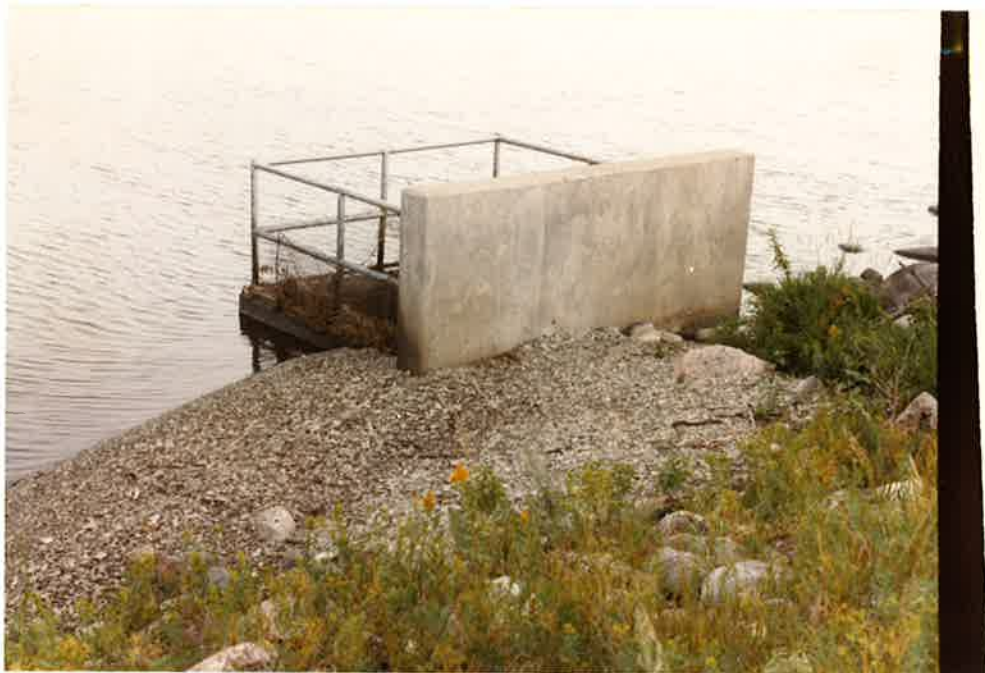
Photo No. 13 - Close-up view of Inlet Structure showing shale deposition on South and East sides of structure.
