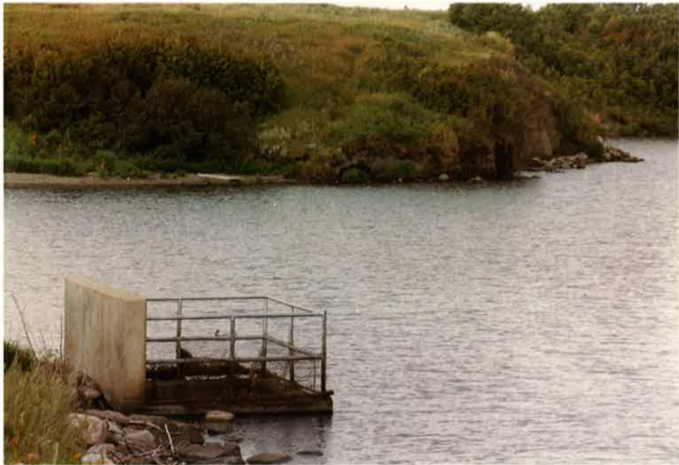
Photo No. 11 - Another view of Inlet Structure and Wave Cut Cliff. Photo taken with telephoto lens.
