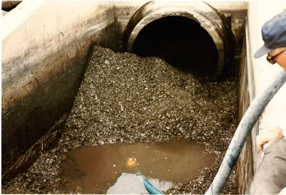
Photo No. 7 - The last of the shale after its removal from the Conduit.
