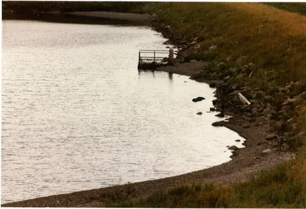
Photo No. 12 - View of Inlet Structure looking North. Note shale dune on South side of structure and along shore line. Another shale dune is exposed to the North of the structure.
