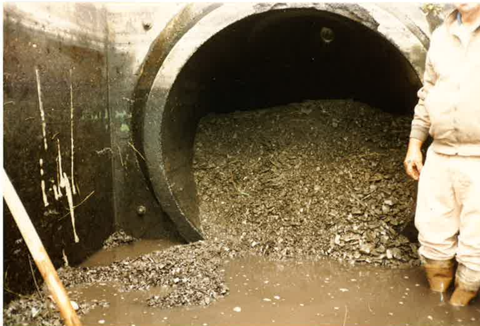
Photo No. 4 - Partial view of Stilling Basin and Conduit. Note shale remaining in Conduit that had to be removed manually.
