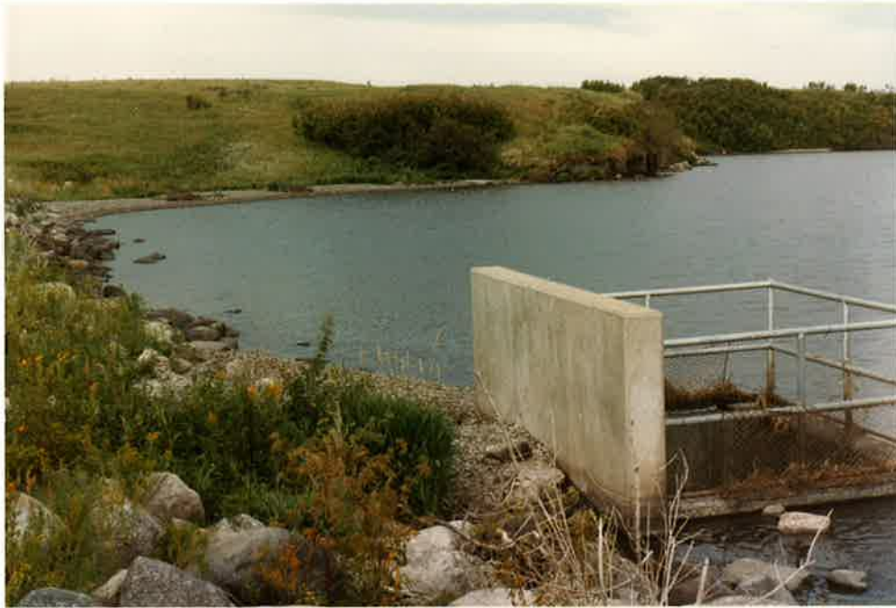
Photo No. 10 - View of Inlet Structure in relation to Wave Cut Cliff. Viewed from the Inlet Structure looking South-westerly towards the cliff.
