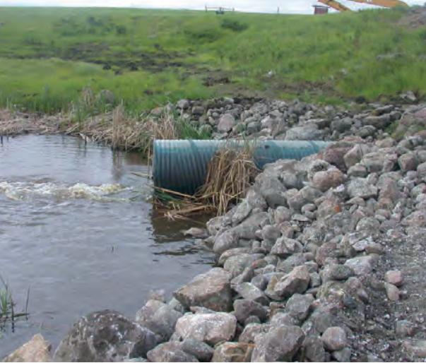
The downstream section of the new corrugated metal pipe spillway at Sarnia Dam.
