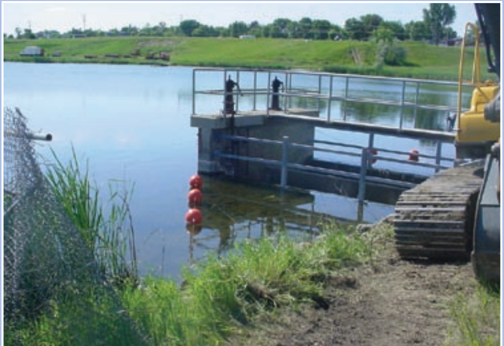
The new steel railing and string buoys around the Harvey Dam drop inlet.
