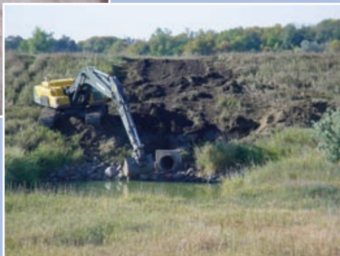
Above: The construction crew makes preparations for the pouring of the concrete cap at Long Creek Dam.
