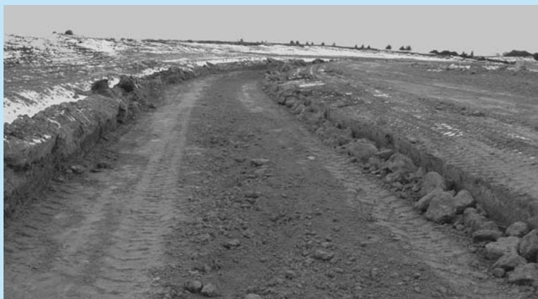
A portion of the open channel construction completed by Park Construction during the Fall of 2003.
